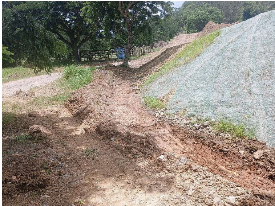
Ditch coming from the west side of the property constructed to divert stormwater flow to outfall 001 from alleged discrete discharge point identified in the EPA inspection report as outfall 002 South side slope of the project with erosion control blanket installed.
