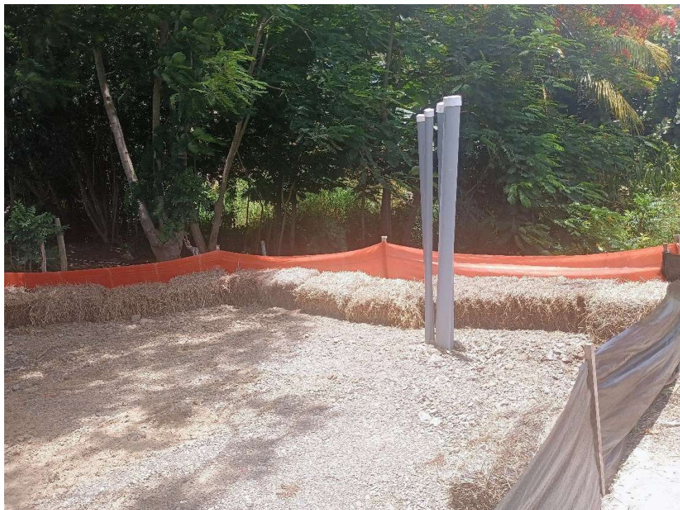
Area located at the south corner of the site identified in the EPA discrete outfall 004 BMPs were implemented in the area (hay bales and silt fence) and it is not a point source as defined in the 2022 CGP permit due to that the stormwater in a sheet (laminar) flow.
